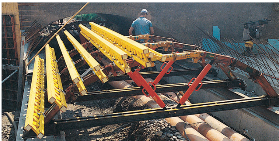
GRV circular formwork and steel walers as self-supporting shoring for arched bridges.
